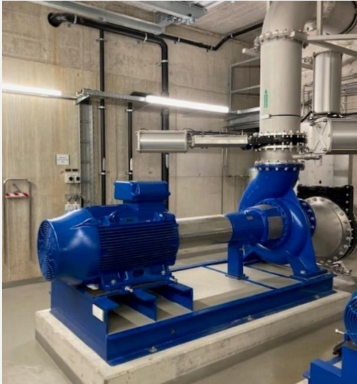
Pumpe EMV-Pumpwerk Morgental
